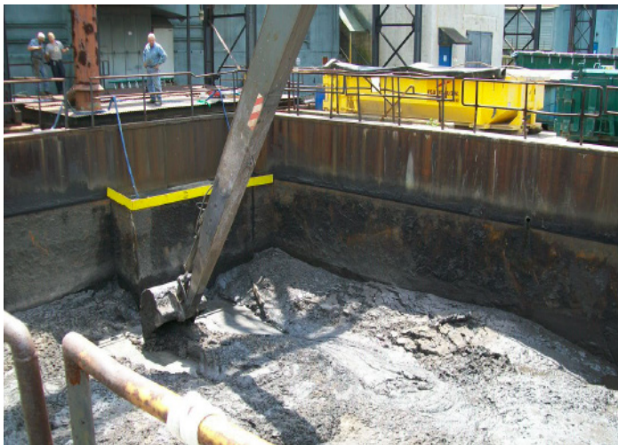
Solidification of WWTP Sludge
